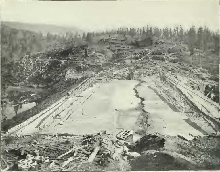
FIG. 1.—CRANE VALLEY DAM, AT A MORE ADVANCED STAGE. THE SLICED EARTH AFTER A FEW DAYS' SETTLEMENT, IS ABLE TO BEAR UP A TEAM ON THE OUTER THIRDS, WHILE THE CENTER IS STILL LIQUID.
