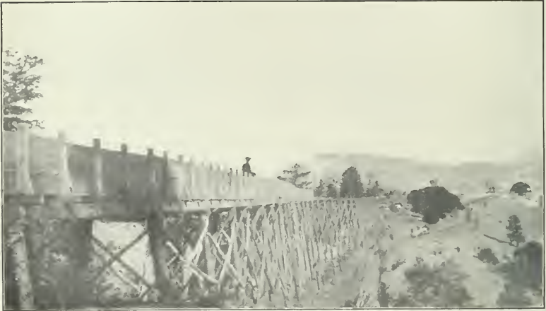
FIG. 1.—FLUME UNDER CONSTRUCTION FOR CARRYING WATER FOR SLICING OPERATIONS ON TERRACE DAM.
