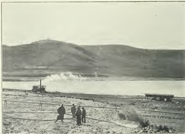
FIG. 2.—SILVER LAKE DAM. LOS ANGELES. THE EARTH, LOOSENED BY THE HYDRAULIC JET, IS CONVEYED TO THE PUMPING STATION SHOWN, AND PUMPED TO THE DAM.
