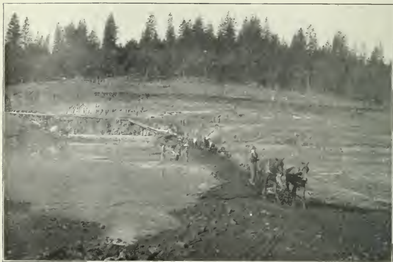
FIG. 1.—LAKE FRANCES DAM, SHOWING DELIVERY OF WATER AND EARTH FROM PIPE ON NORTH FACE.
