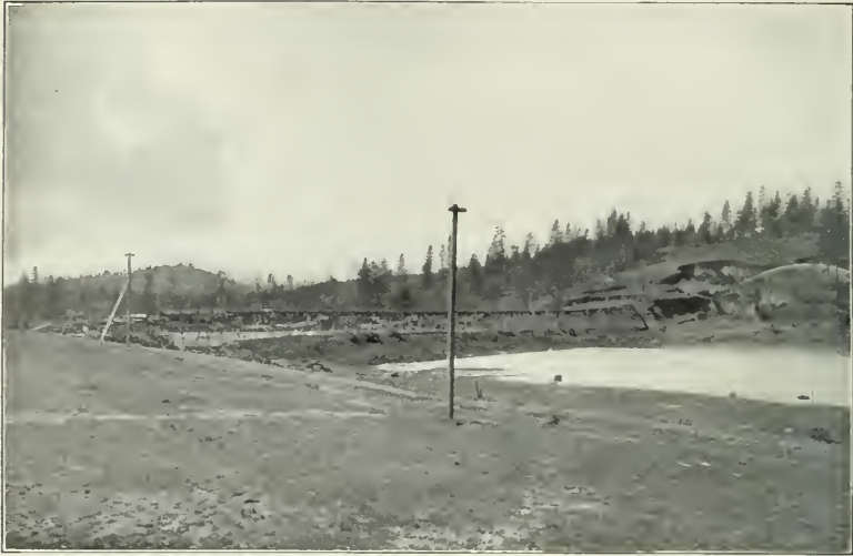
FIG. 1.—LAKE FRANCES DAM FROM THE EAST END. SHOWING FINAL TRESTLE AND SLUICE PIPE, AND GENERAL VIEW OF BORROW-PIT.
