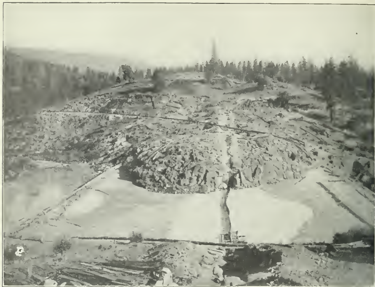
FIG. 1.—CRANE VALLEY DAM. SHOWING WOODEN FENCE, OR CENTER DIAPHRAGM, WHICH WAS CARRIED UP TO A HEIGHT OF 30 FT. ABOVE BED-ROCK.
