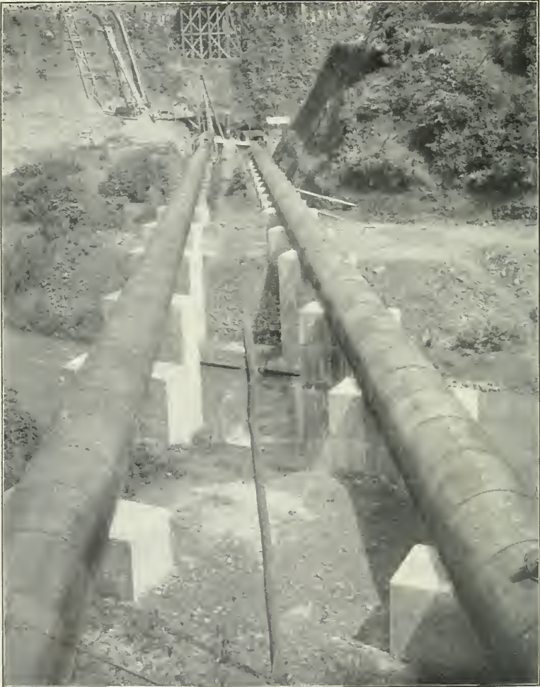
PIPE LINES FROM TUNNEL NO. 5.
