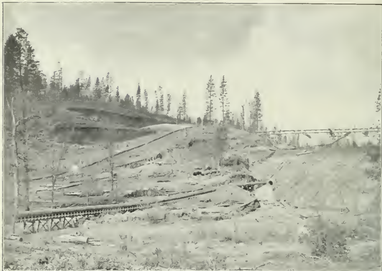
FIG. 1.—WEST END OF LAKE FRANCES DAM, SHOWING THE BREAK RESTORED, THE HIGHER DAM NEARLY COMPLETED, THE HYDRAULIC GIANT AT WORK, AND THE MAIN PIPE LINE SUPPLYING WATER TO THE PUMP.
