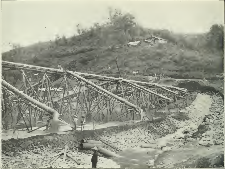
FIG. 1.—LIQUID EARTH BEING DEPOSITED THROUGH PIPES ON OUTER SLOPES OF DAM No. 1, TENANGO RIVER.
