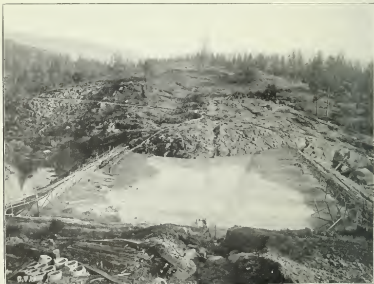
FIG. 2.—CRANE VALLEY DAM, SHOWING DISCHARGE OF SLUCED EARTH AT END OF CONVEYING FLUME.
