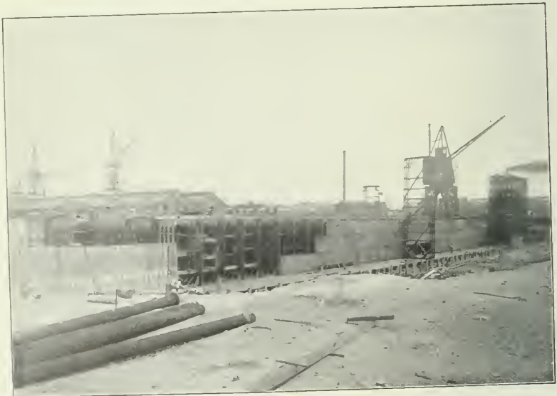
FIG. 2.—VIEW OF DOCK, MARCH 16TH, 1904, SHOWING BOTTOM PLATING IN PLACE ON BLOCKING IN BUILDING BASIN. MAIN PONTOON FRAMING, ETC.
