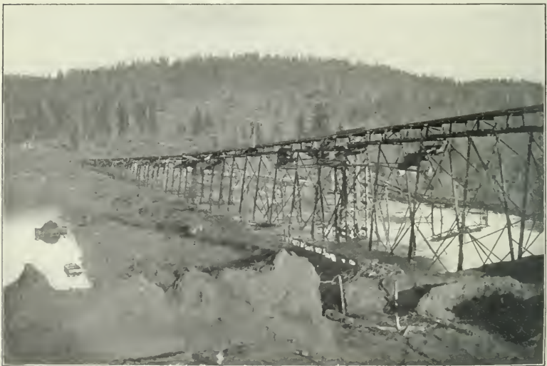
FIG. 2.—LOOKING EAST ALONG LAKE FRANCES DAM. SHOWING OPERATION OF BUILDING UP SLOPES WITH BRUSH.
