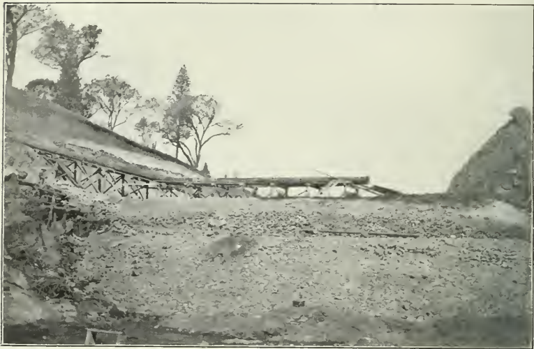
FIG. 1.—LAKE FRANCES DAM. LOWER FACE OF DAM AT BREAK, RIP-RAPPED WITH ROCK.
