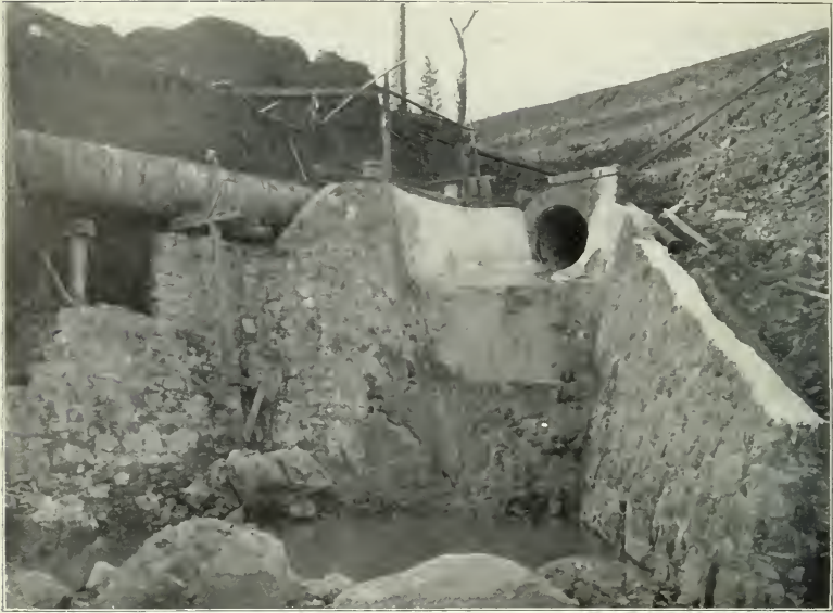
FIG. 1.—LAKE FRANCES DAM. DISCHARGE END OF WASTEWAY OUTLET CULVERT, USED AS AUXILIARY TO MAIN SPILLWAY FOR EMERGENCY RELIEF.
