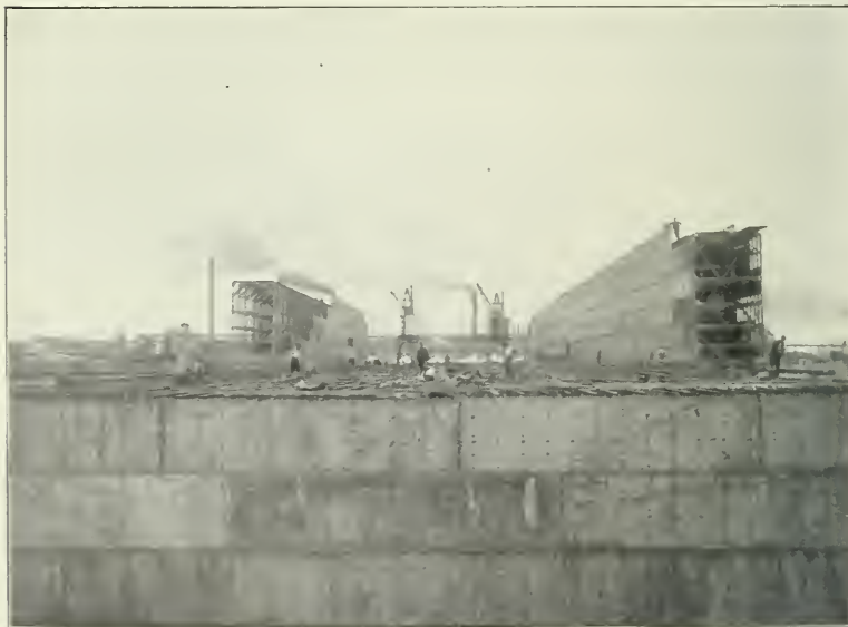
FIG. 2.—VIEW OF DOCK, AUGUST 1ST, 1904, SHOWING SKIN PLATING OF PONTOONS AND SIDE WALLS.
