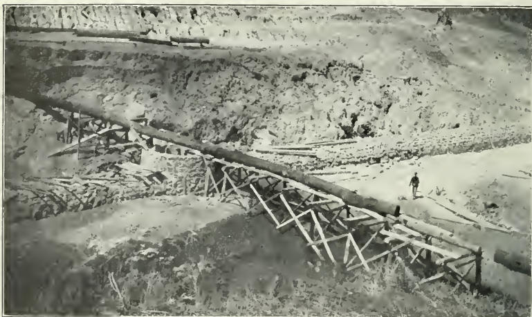
FIG. 1.—LAKE FRANCES DAM. SLUICE PIPE ALONG INNER TOE OF ORIGINAL DAM, FOR DEPOSITING COARSE, POROUS MATERIAL.
