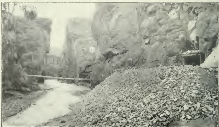
FIG. 2.—LOOKING UP STREAM THROUGH THE GORGE IN WHICH THE TERRACE DAM IS BEING BUILT,
