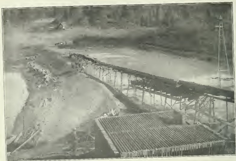
FIG. 1.—TOE LEVEE OF NORTH FACE, LAKE FRANCES DAM, AND INLET CRIB AT HEAD OF SIX-FOOT OUTLET CULVERT.
