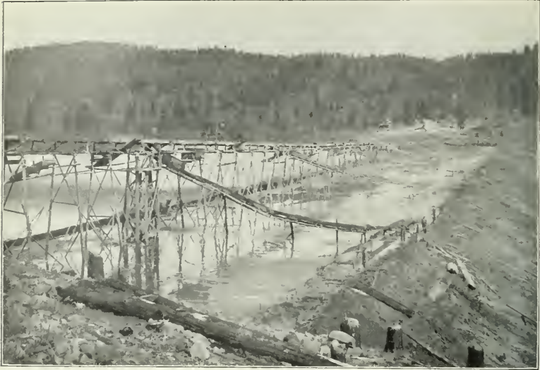
FIG. 1.—HYDRAULIC-FILL DAM BUILDING, SHOWING OUTER LEVEES MAINTAINED WITH BRUSH, DEFLECTING BOARDS FOR DISTRIBUTING SLICINGS ALONG SLOPE. GENTLE SLOPES TOWARD CENTER OF DAM, AND GRADUAL MOVEMENT OF DRAINAGE TOWARD EXTREME END.
