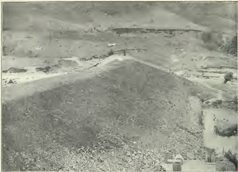
FIG. 1.—DAM No. 1, TENANGO RIVER. THE MATERIALS FOR THE DAM WERE GROUND-SLICED FROM THE BORROW-PITS IN THE BACKGROUND.
