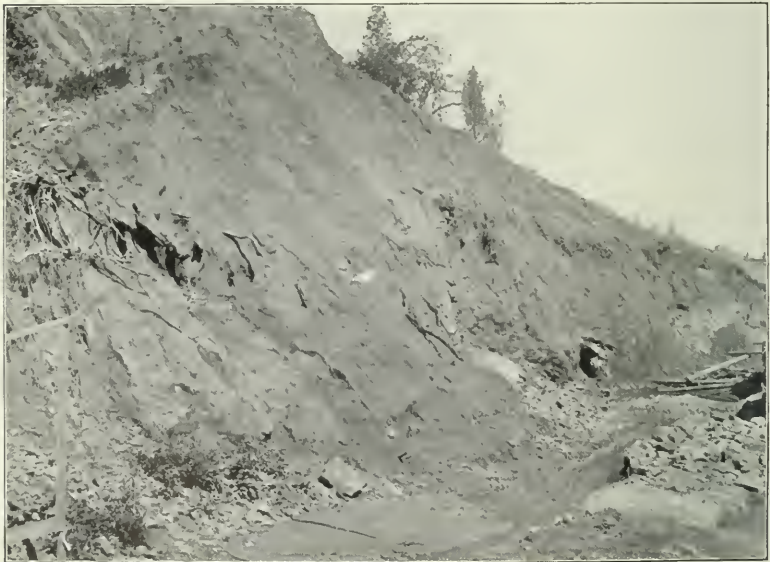
FIG. 2.—NEAR VIEW OF RIGHT SIDE OF BREAK IN EMBANKMENT OF LAKE FRANCES DAM, SHOWING ROOTS EXPOSED BY THE BREAK.
