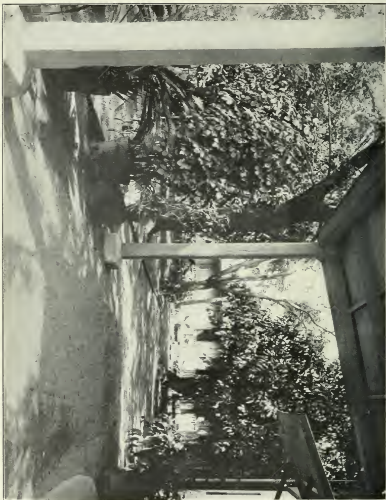
PORCH OF RESIDENCE IN MANILA, SHOWING CRACK IN POST ATTACKED BY WHITE ANTS.
