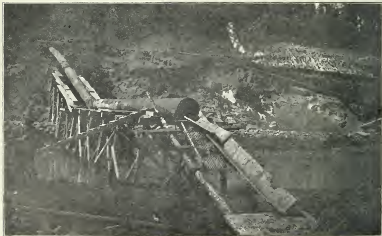
FIG. 2.—LAKE FRANCES DAM. SLUICE PIPE USED WITH SIX-INCH PUMP, SHOWING GRIZZLY AT END.
